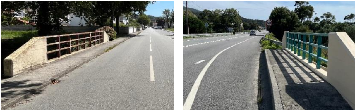
Figure 3. Example of maintenance conditions of contemporary (and same type) bridges on secondary local (left) and national (right) roads.
